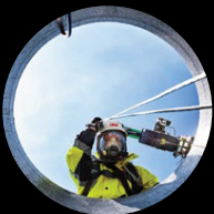
Outdoor or Underground
